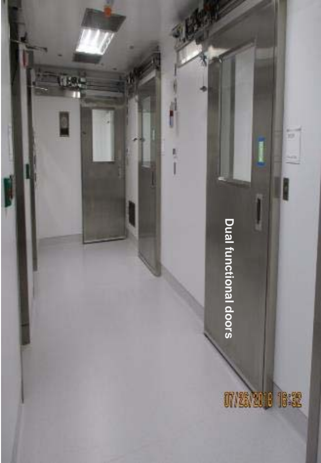
vestibule to the clean room suites
